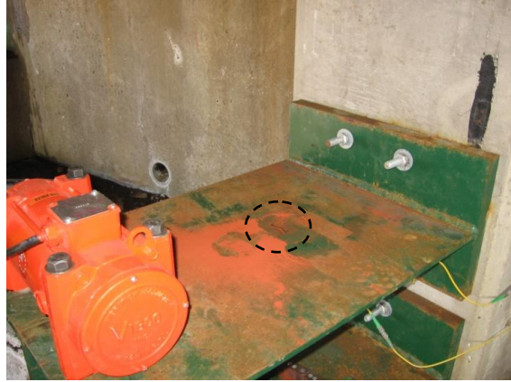
a. Overview of Top Web-Plate Cracking
