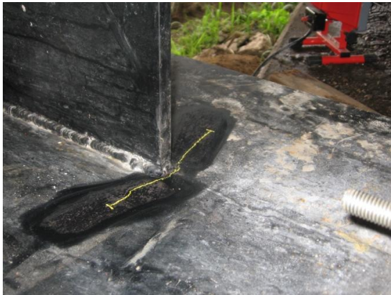
c. Bottom web plate cracking
