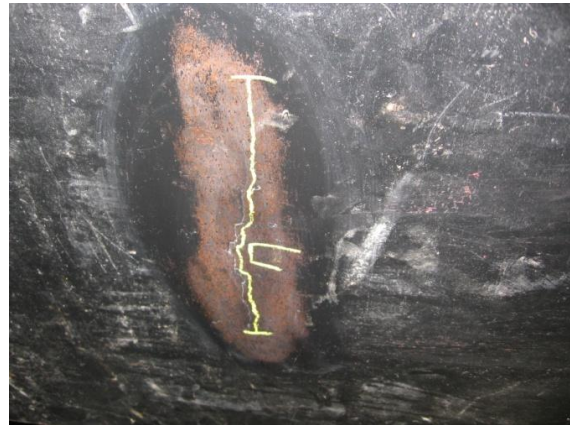
d. Underside of bottom web plate cracking
