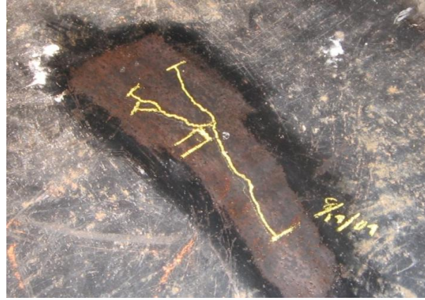
b. Close-up of top web plate cracking
